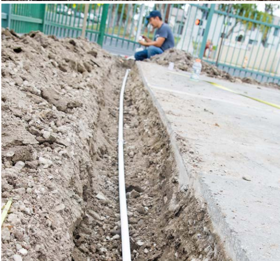
Above, from top to bottom. Cutting Asphalt; Rototilling the Soil; Installing Irrigation
